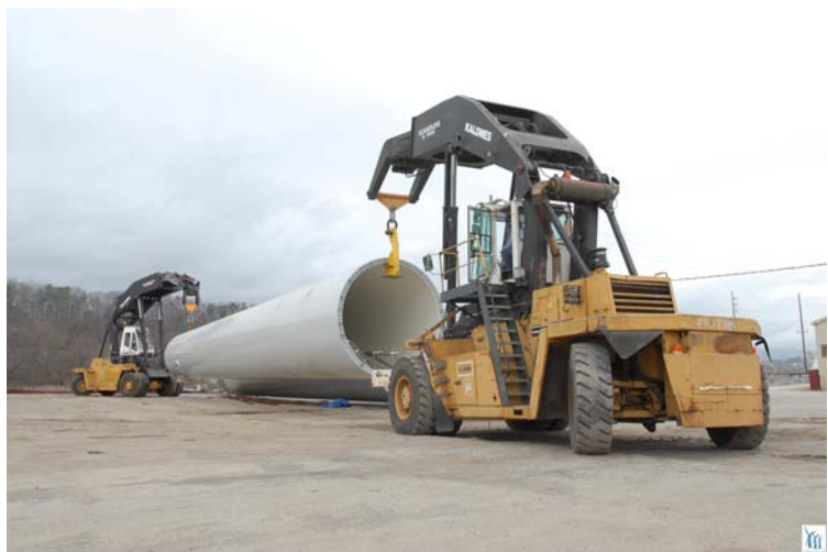
Construction at a wind project in Chattanooga, Tennessee. Photo courtesy of AWEA.
