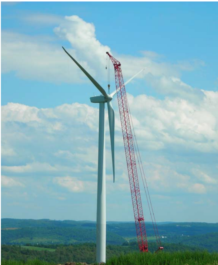
Erecting a wind turbine at the Munnsville Wind Power Project. Photo courtesy of AWEA.
