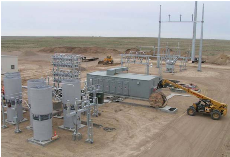
Construction of a substation at the Big Horn Wind Project in Klickitat County, Washington. Photo courtesy of PPM Energy.
