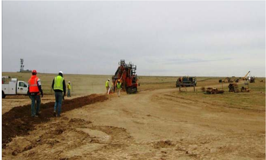
Construction personnel trenching for an underground collector cable. Photo courtesy of PPM Energy.
